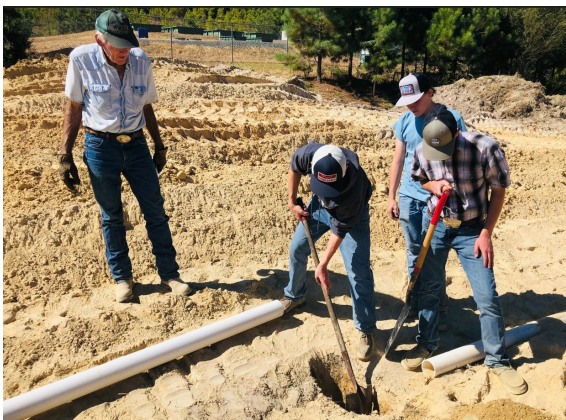
Don Youngblood gets some assistance constructing the wetland pond by students of Cossatot River High School
